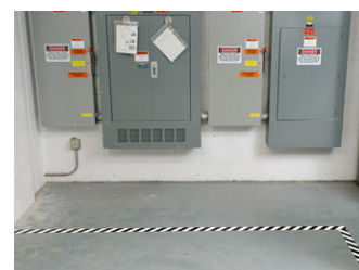
6. Colour-code areas in front of electrical panels.
